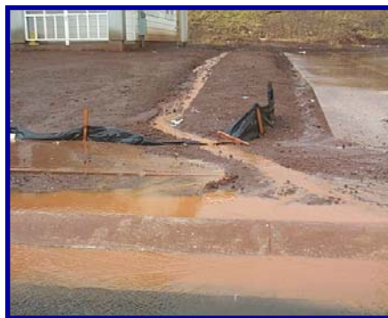
Soil erosion during construction
