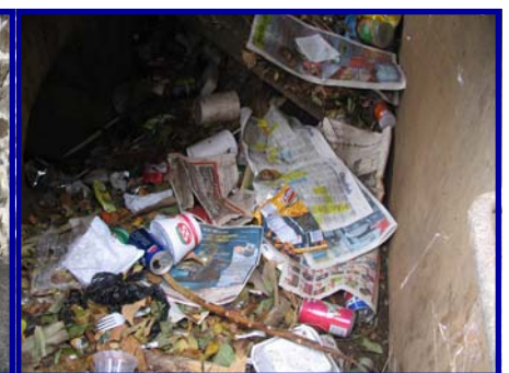
Trash inside a catch basin
